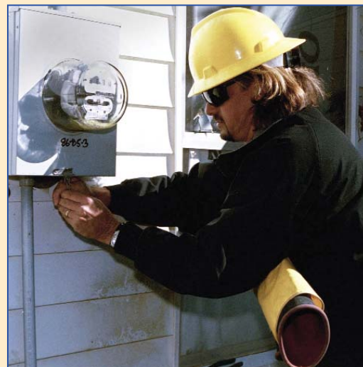
Barry McGarva re-seals a meter after making sure it is working properly.
