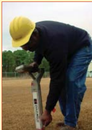
Melvin Davis, CCEC operations technician and materials handler, uses a device to find and mark underground power lines before digging nearby.
