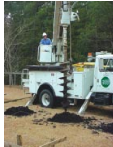
Crew Leader Paul Quillen drills holes in order to set 16-foot posts.
