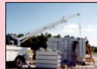
New substations meet the needs projected by Engineering personel.
