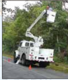
A retired CCEC bucket truck is used in the field by “sister” co-op Cooperativa Eléctrica del los Santos in Costa Rica.
